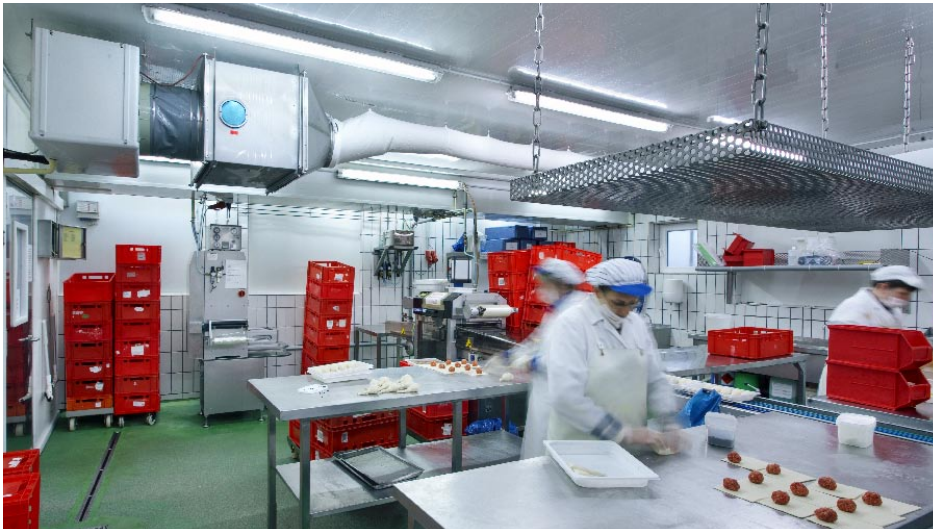
Two UV-C disinfection systems positioned as evaporator series connection units turn the meat preparation area into a bacteria-free zone.
